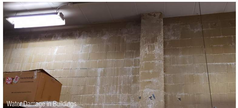
Water Damage in Buildings
